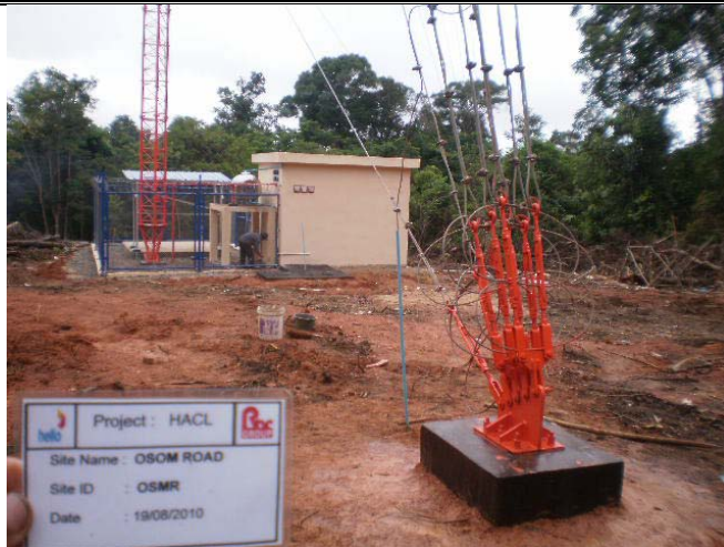
Tower Connecting to Grounding System(3)
