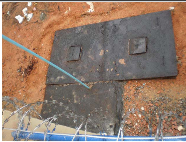
Sewage System & Septic Tank
