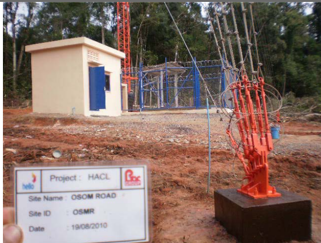
Tower Connecting to Grounding System(2)
