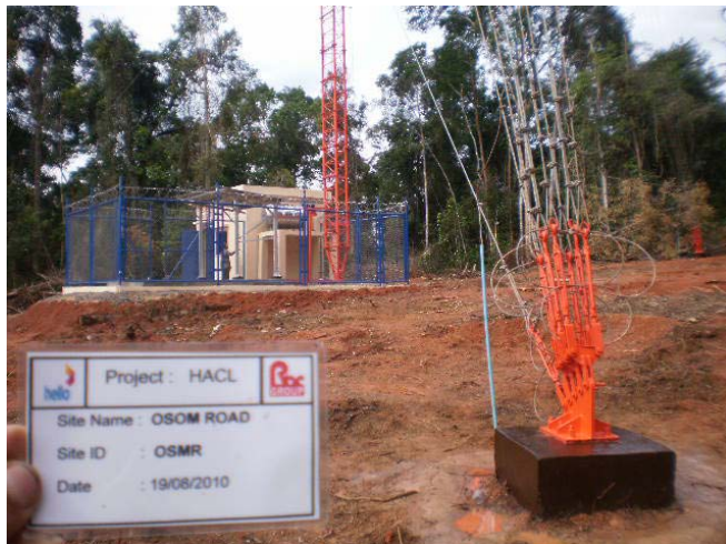
Tower Connecting to Grounding System(1)
